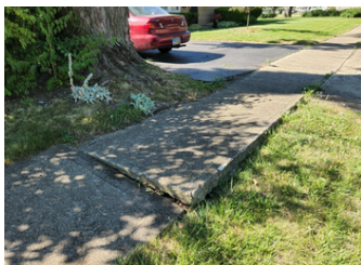
Tree damage - Resident Responsible
