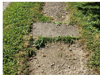
Disintegrated Sidewalk - Resident Responsible
