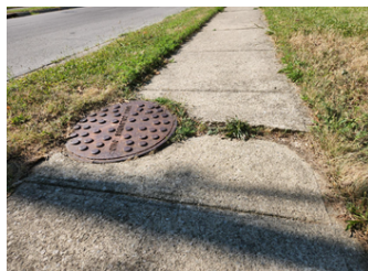
Crack Utility Defect - City Responsible
