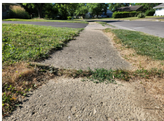
Vertical Separation Defect - Resident Responsible
