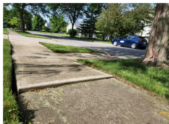
Vertical Separation - Tree damage - City Responsible
