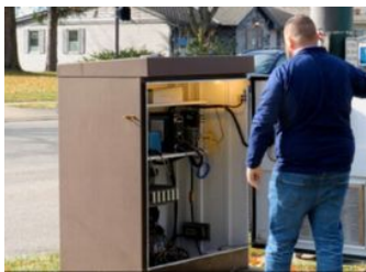
Traffic Signal Control Box
